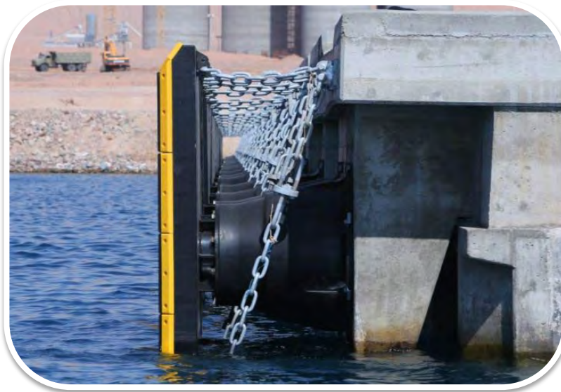
Dock face with modern fenders
