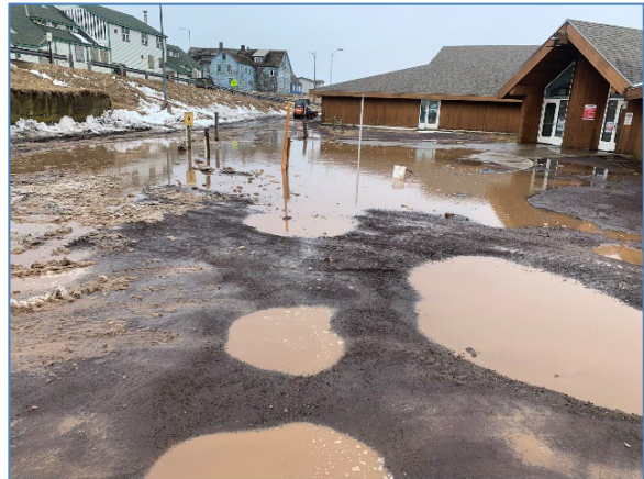
Lack of delineation and unsafe road conditions in front of School drop off area.
