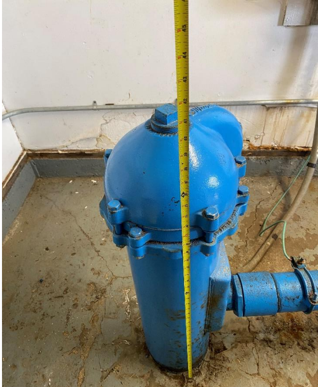
Photo 9: North well casing 31 inches above floor.
