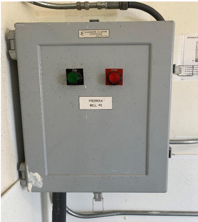
Photo 41: Fredrika well #5 electrical box.
