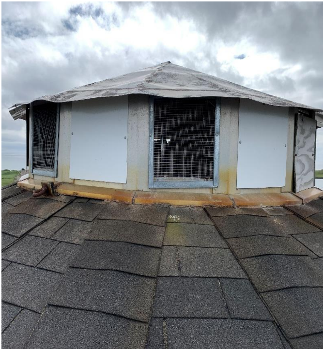
Photo 54: Top of WST 2 screened.
