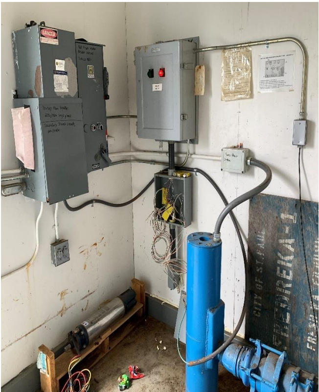
Photo 19: Electrical control boxes.
