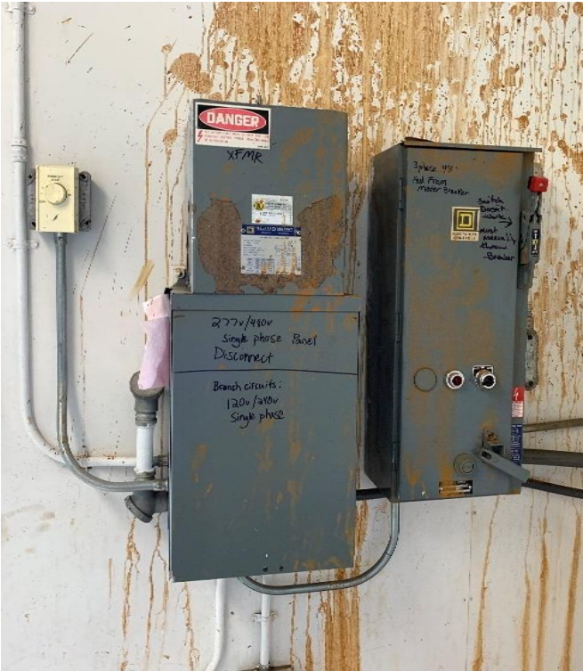
Photo 26: Electrical control boxes.
