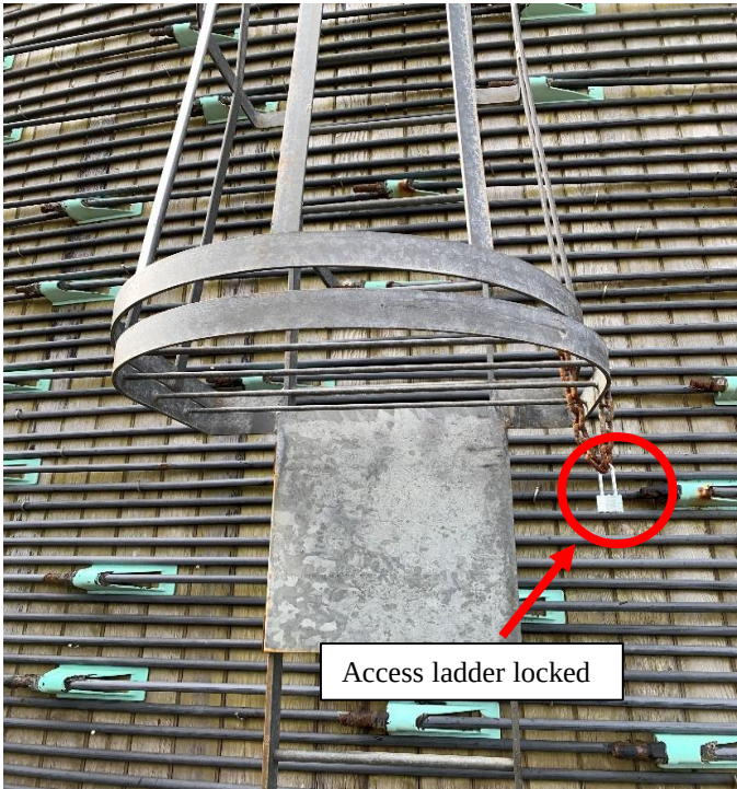
Photo 53: Access ladder locked on WST 1.
