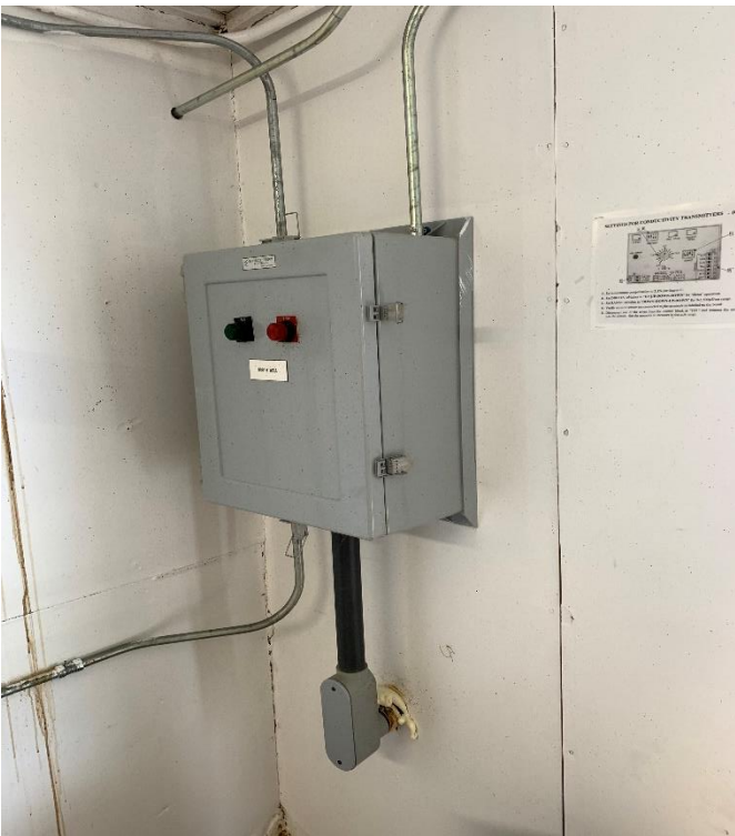
Photo 15: North well electrical control panel.
