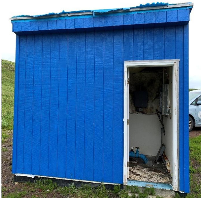
Photo 35: Well house exterior, roof in disrepair.
