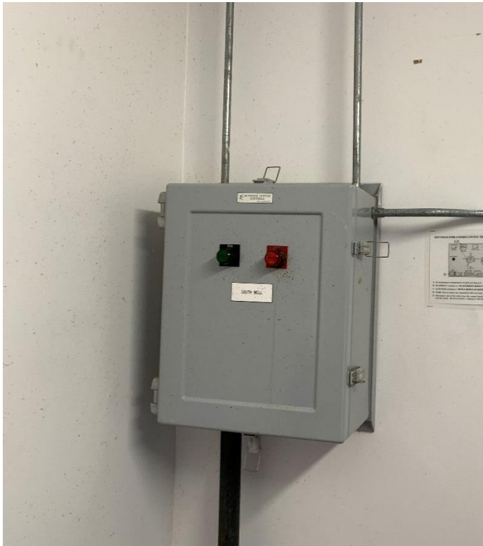
Photo 3: South well control panel.
