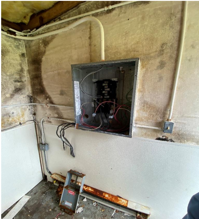
Photo 37: Well house electrical control panels disabled.
