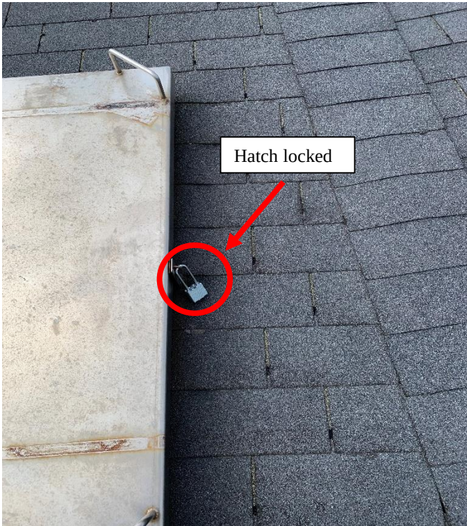
Photo 52: Hatch locked on WST 1.
