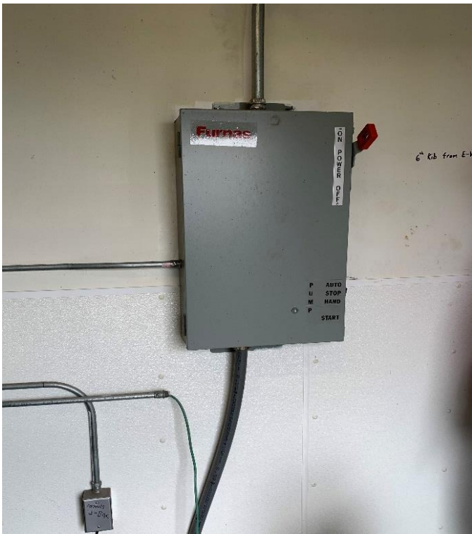
Photo 42: Fredrika well #5 pump control electrical box.
