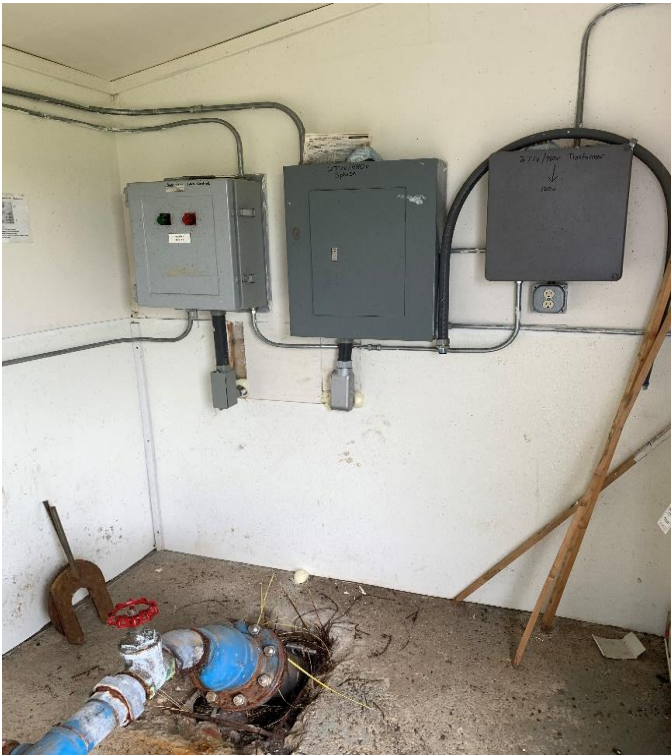
Photo 32: Well house electrical control panels.
