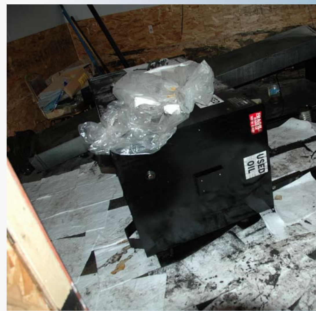
Used oil container toppled during flood; it could be elevated and anchored.
